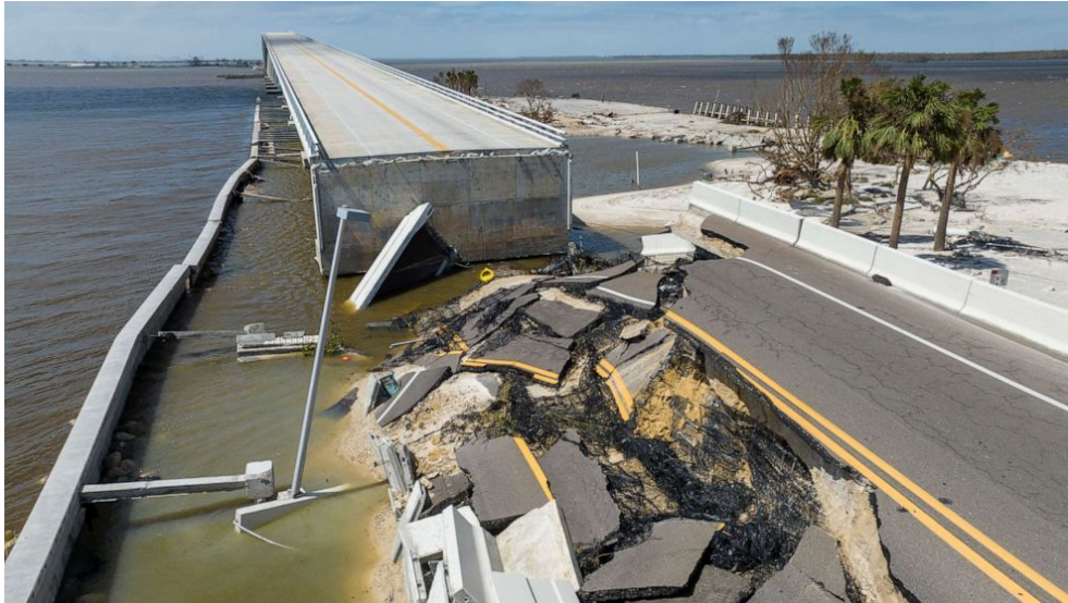
A section of the Sanibel Causeway that was washed away by Hurricane Ian, Sept. 29, 2022, in Fort Meyers, Fla.
